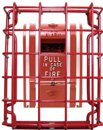
Guard pictured with Edwards Systems Technology SIGA-270 Fire Alarm
